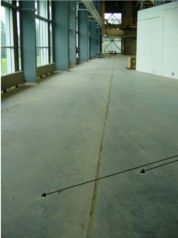
Jointed floor to stop wind on building shell affecting storage ring (CLS) (300 mm slab on thick glacial till)
